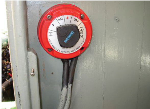
A faulty battery switch and the result of no action being taken
